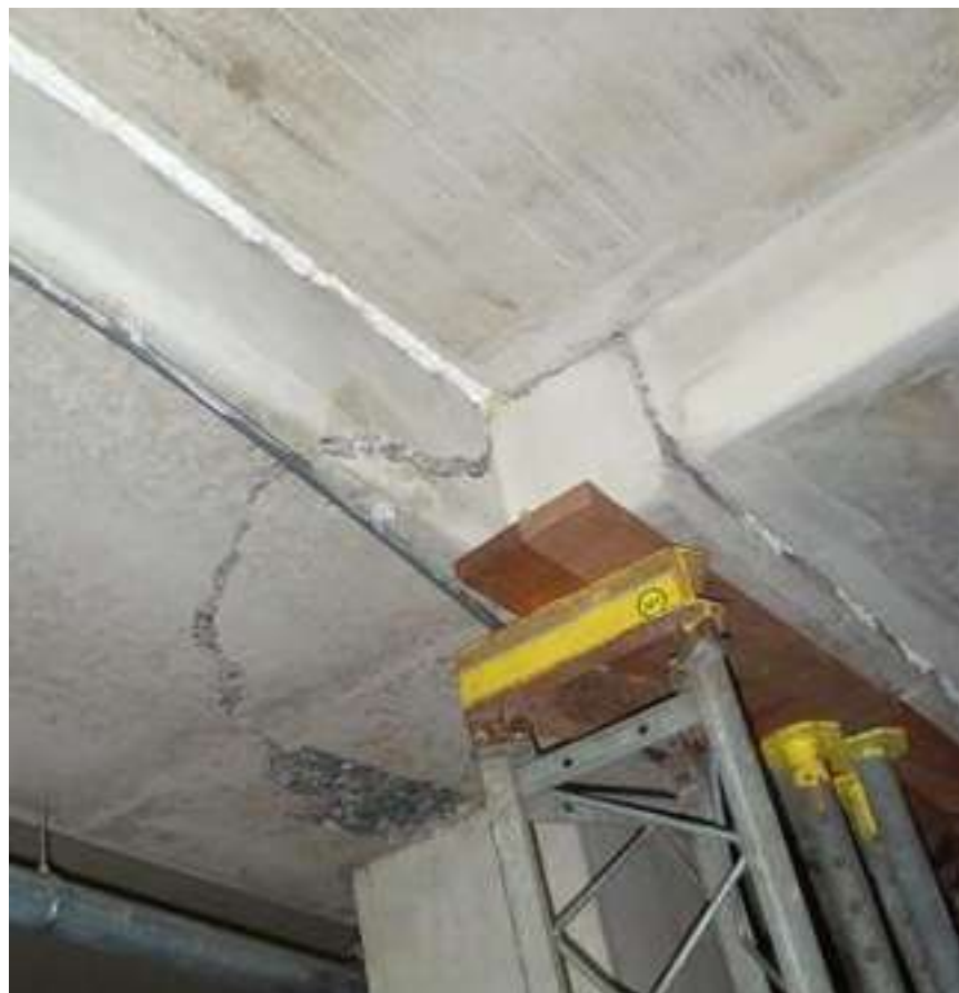
Foto 2.6: Afgebroken nok op as 11, stramien J
